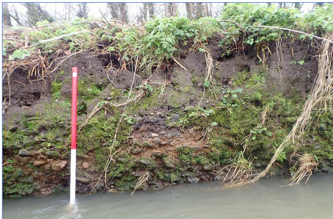
Plate 13: South bank at the upstream end of the required survey area, showing a humic topsoil over gravel till.
