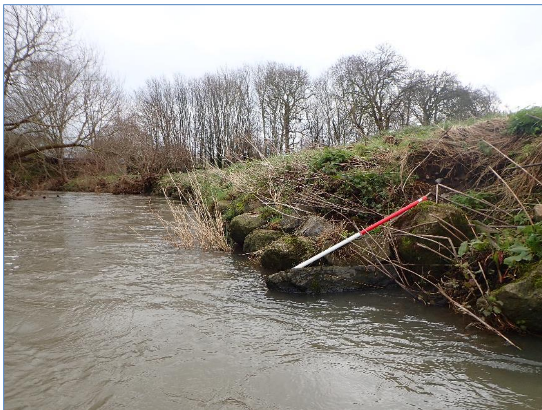
Plate 14: Upstream limit of the second expanse of rock armour protection to the south bank.
