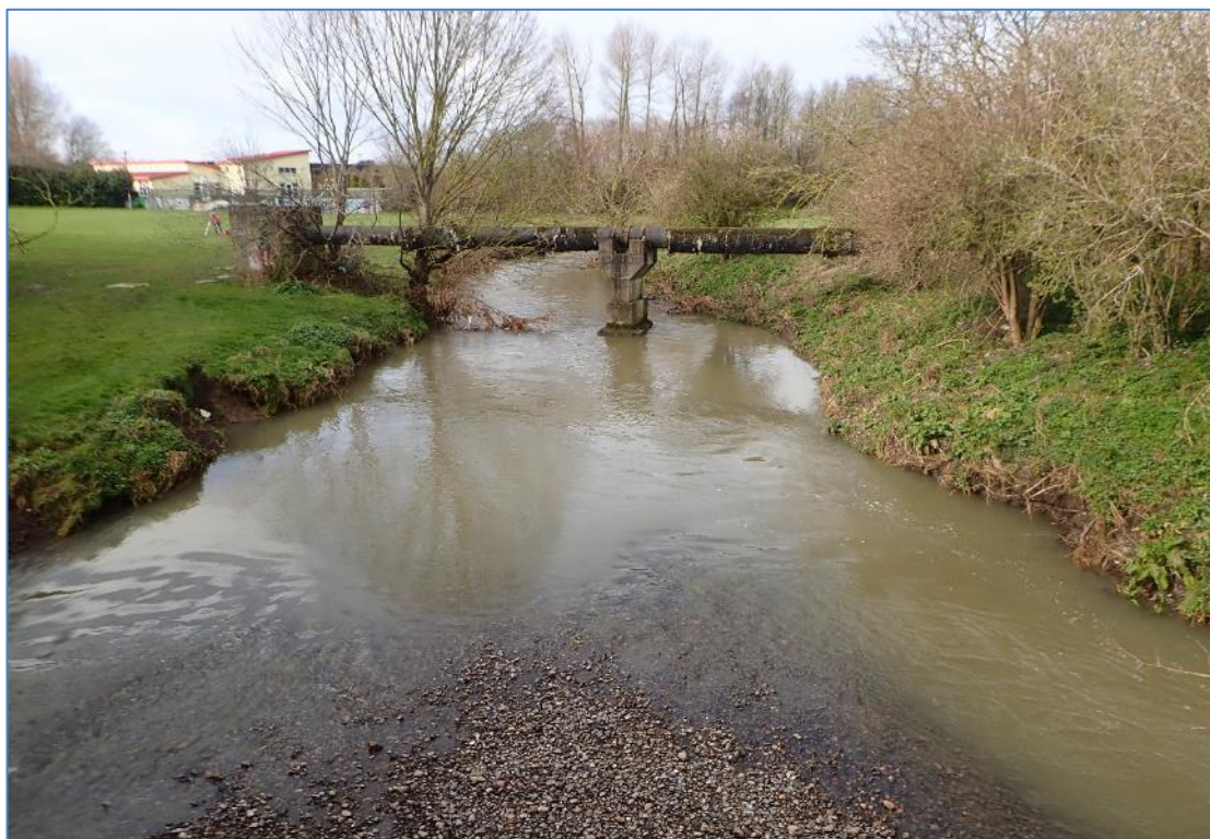
Plate 10: The services pipe that crosses the Broadmeadow River at the downstream end of the survey area. View from Lissenhall Bridge.
